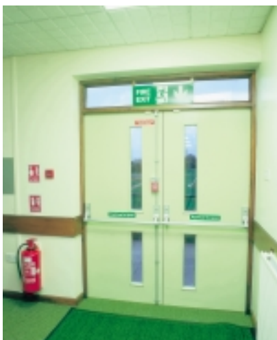
Fire exit push bar, break glass call point, exit sign & water extinguisher.
